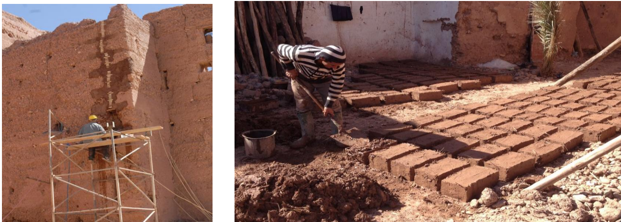
Figure 4 – Conservation works in the Stara, including repairing a structural crack (left), and preparation of adobe bricks (right). Photos: Benjamin Marcus, 2014.
