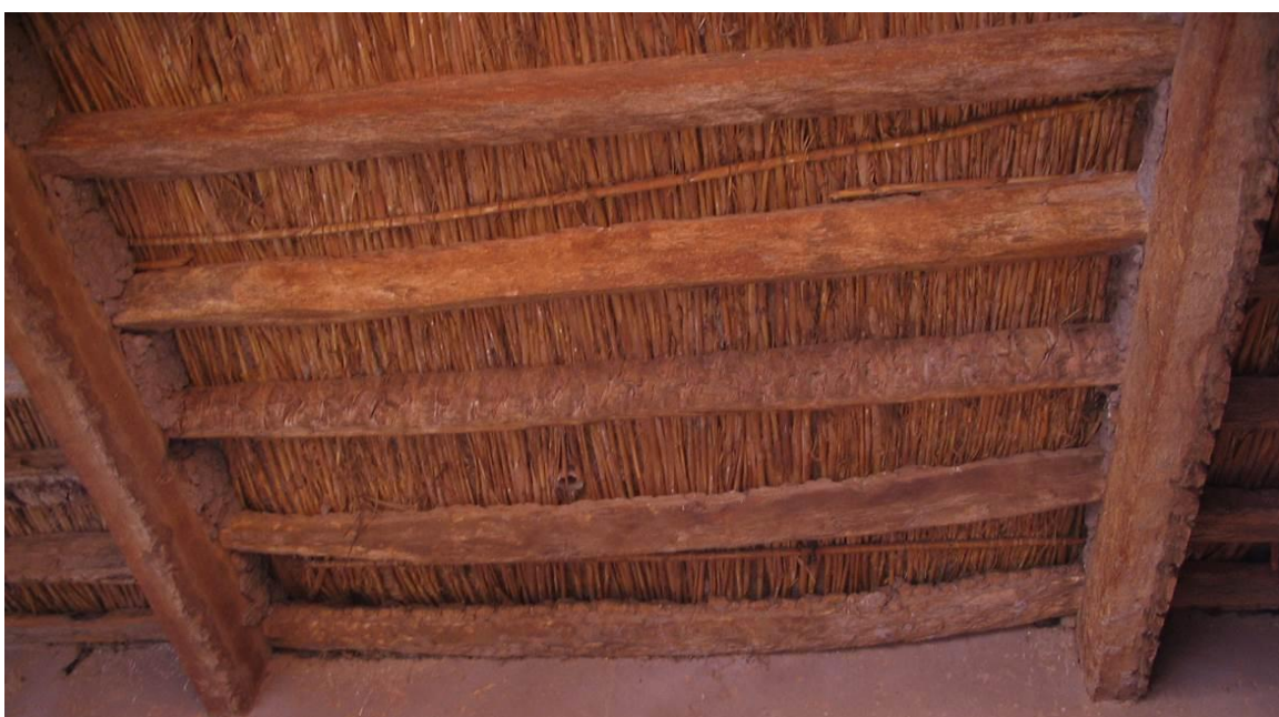
Figure 10: Example of horizontal structure made with palm wood and a layer of canes.
