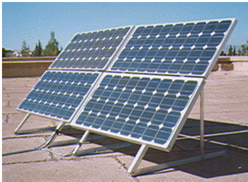
Figure 5: PV panels installed in the laboratory.
