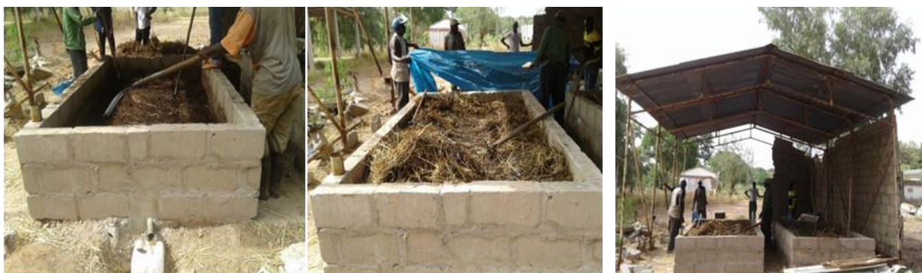
Figure 1: composting units with shelters
