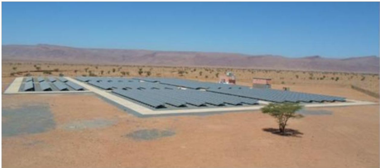
Figure 1: View of the 806.52 kWp grid-connected PV system installed at the Assa Town, southern Morocco.
